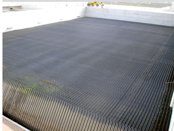
Figure 4: Lamella clarification filter
